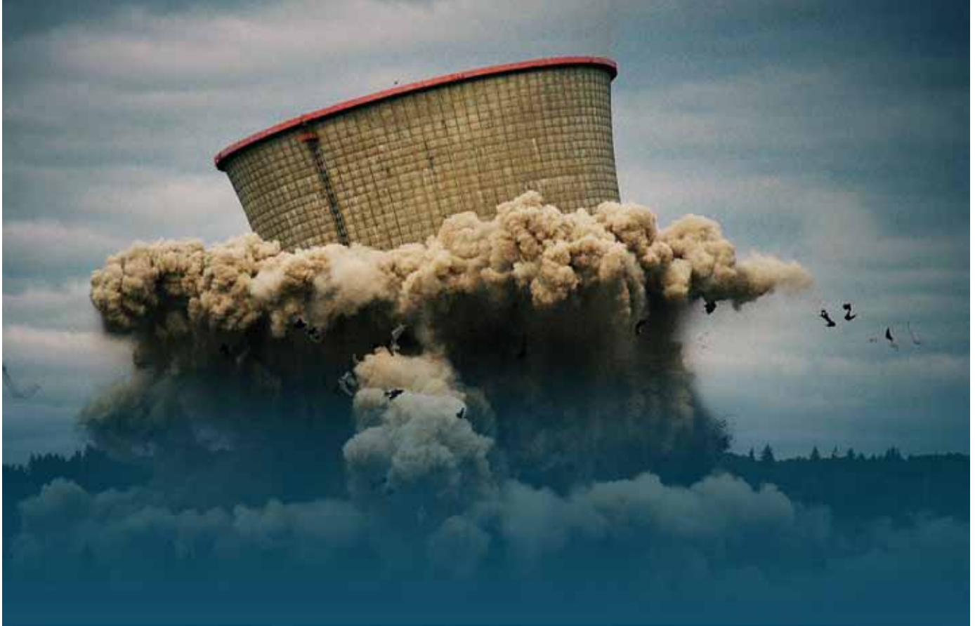
Decommissioning of the cooling tower of the Trojan nuclear power plant, Oregon, USA, May 2006.
