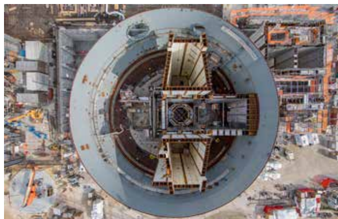
One of the two long-delayed, over-budget AP1000 reactors under construction in Georgia, USA.
