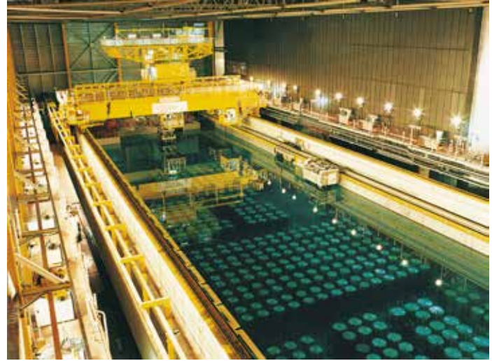
THORP reprocessing plant.
